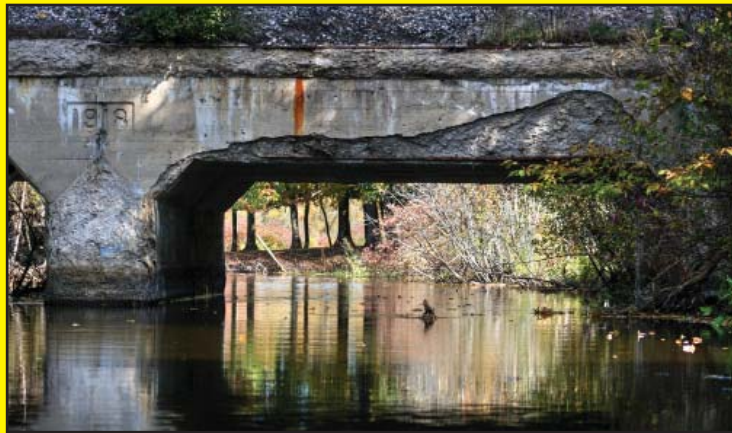
The 1918 Railroad Bridge over the Grand River running alongside the Brooklyn Highway
